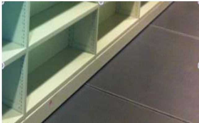
The floor panels are supported by mobile rails that form a solid platform that do not require fixing to the existing floor.
